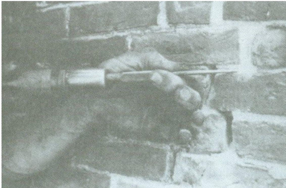
Operator using \frac{3}{4} "-D Tool with \frac{1}{8} " Cape Chisel on Mortar Joint
